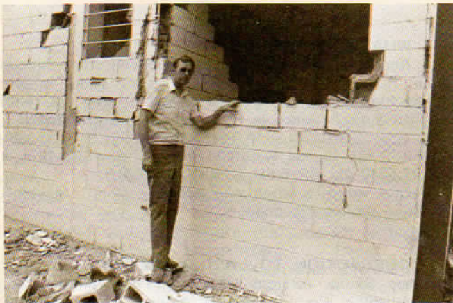
Quake damage to Radio Station HCRI, Santa Rosa
